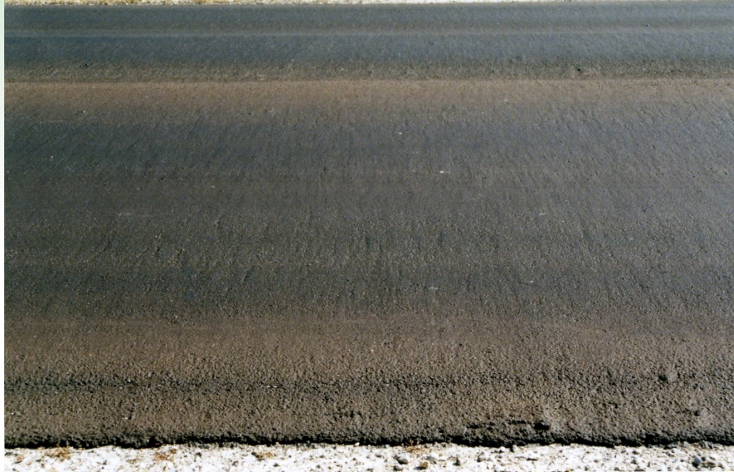
Poor Construction and Quality Control
