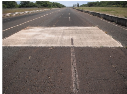
Figure 2 – Existing Track Condition: Concrete patches along track length.
