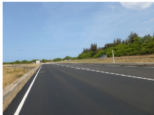
Figure 8 – AC pavement joints kept at mid-lane to minimize impact of vehicle tires.
