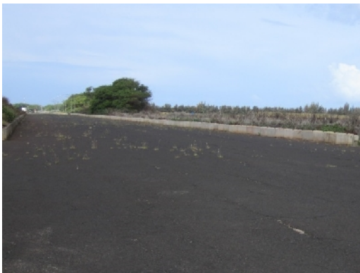
Figure 1 – Existing Track Condition: Grass/Weeds growing through numerous cracks.
