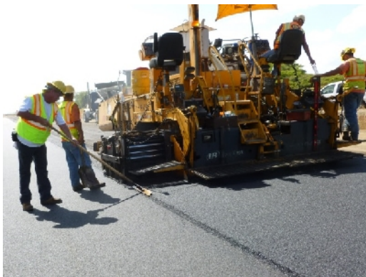
Figure 7 – Good practices result in a good product. Contractor cleans the edge of the pavement joints before rolling.
